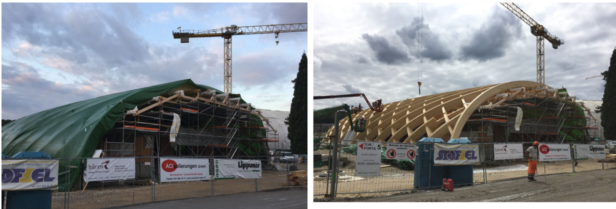
Figure 67: Efficient protection during evenings, nights and weekends or during rain; removing of the protection during the working times (Swatch building, Biel/Bienne)
